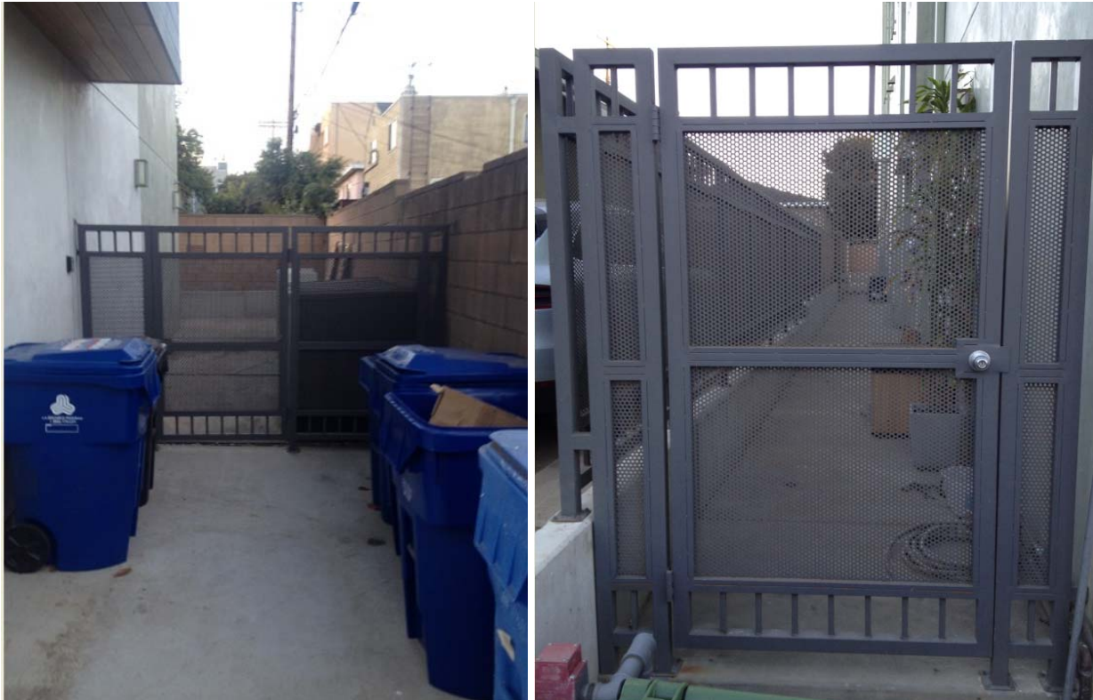
Missouri/Stoner: 10-ft rear yard (no grassy play area) 5-ft. side yard (all concrete, no trees)
